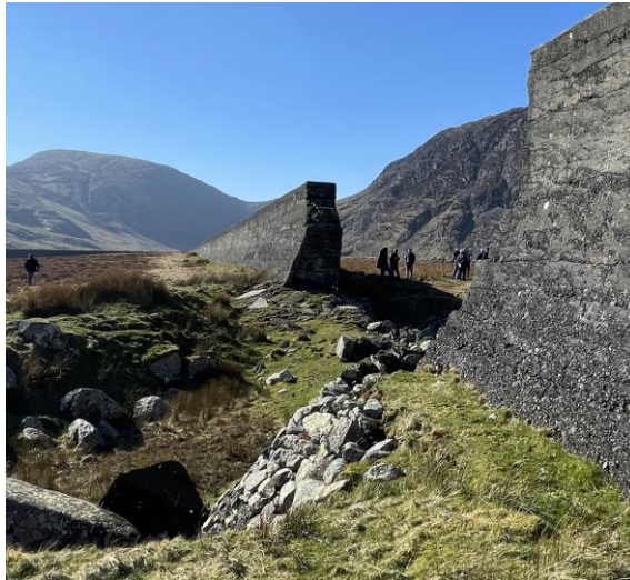
Eigiau Dam, Wales, failed in 1925
